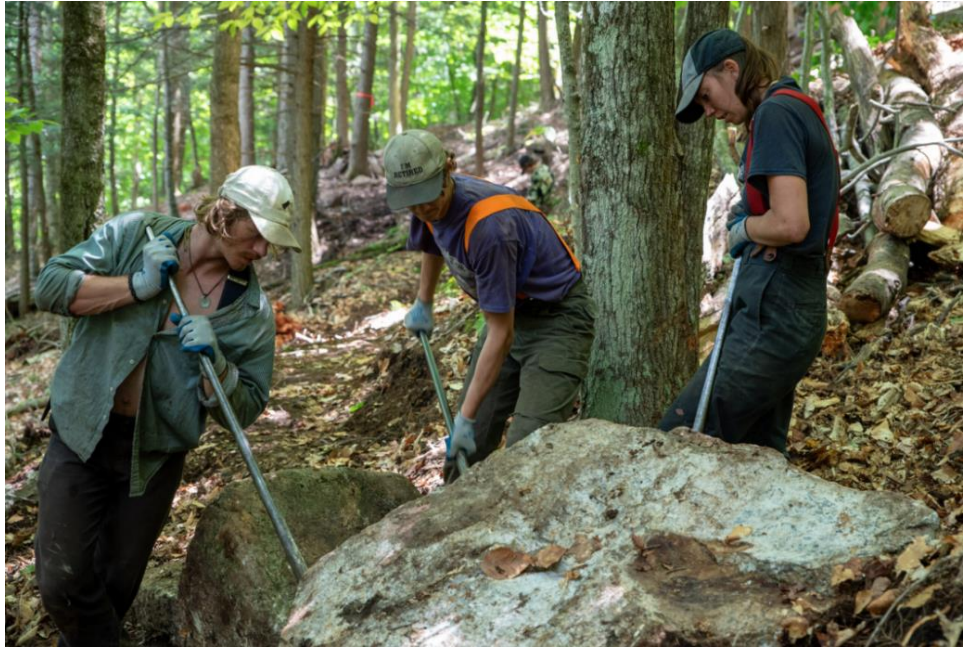
Members of the Pro Crew work on Jones Hill in the Hoffman Notch Wilderness
